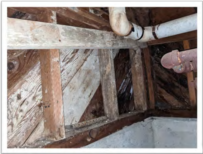
Sample 22-082A.92, Pipe Insulation, 14% Asbestos
