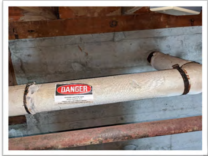
Sample 22-082A.91, Pipe Insulation, 80% Asbestos
