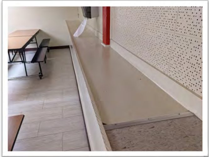
Sample 22-082A.76, Sheet Vinyl, 12% Asbestos
