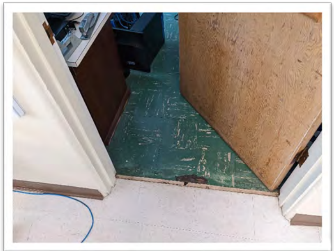
Sample 22-082A.17, Tile/Mastic, 3%/2% Asbestos Sample 22-082A.18, Tile/Mastic, ND/5% Asbestos
